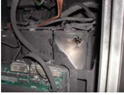
Picture 2: Short-circuiting on the capacitor
